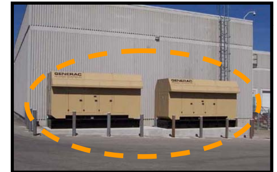
(1). Use of a screening wall in a similar color to the façade would better screen the generator.
