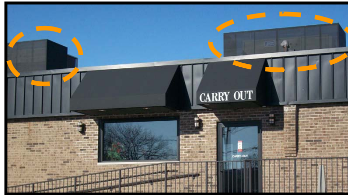
(1). Mechanical units are screened from the view of the parking lot using awning fabric to blend with the mansard roof.
