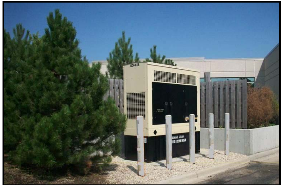
A good example of mechanical equipment being screened year-round by evergreen plantings and solid fencing. It is protected from vehicles by concrete bollards and vents away from the landscaping to protect the plants.
