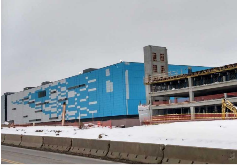
Amazon’s massive terminal facility at CVG, shown here on February 14, 2021, is designed to allow sorting on seven levels and projected to open this year.
